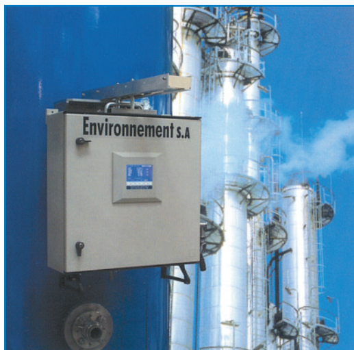
Direct stack installation at refinery
